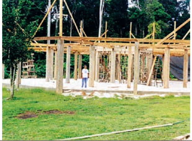
A forest station in the Iwokrama forest, Guyana, built using green-building principles. Photo: Iwokrama International Center
